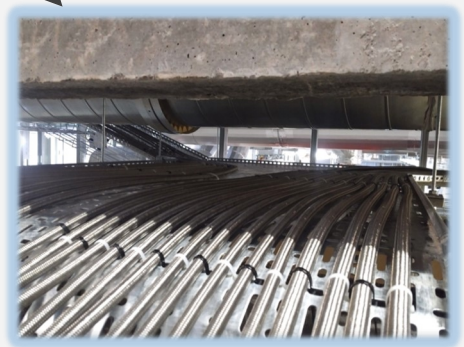
Virgin PTFE hoses installed on stainless steel trays throughout the manufacturing plant.
