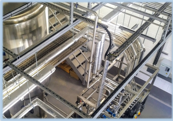
Top view showing virgin PTFE hoses leaving the plant room.
