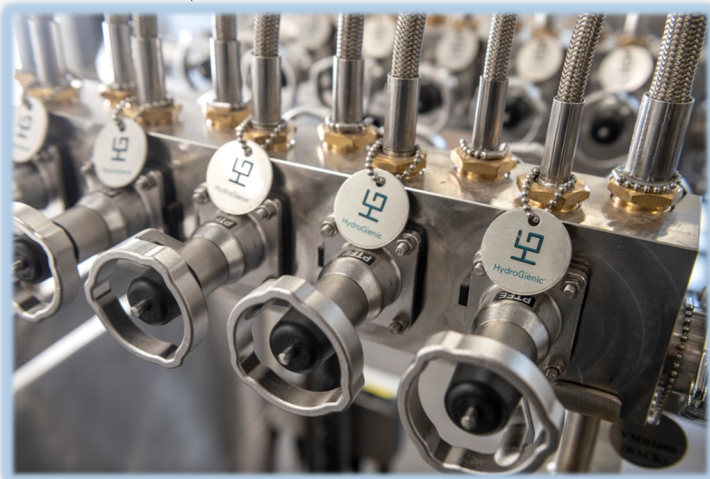
Stainless steel manifold with outgoing flow to offtakes.
