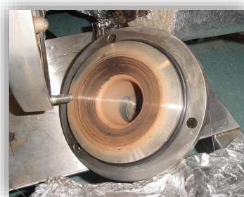
Figure 10 Example of 'rouge' found in a pump casing
