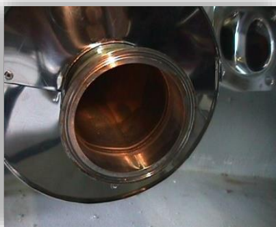
Figure 13 Rouge inside a pipe bore
