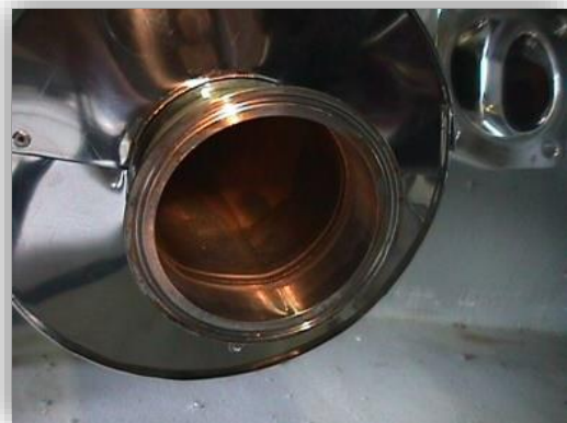
Figure 4 Rouge inside a pipe bore
