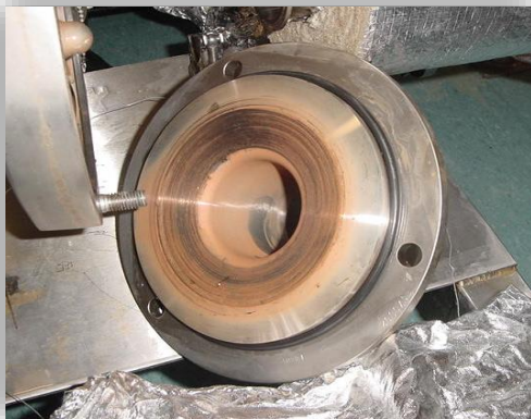
Figure 1 Example of 'rouge' found in a pump casing
