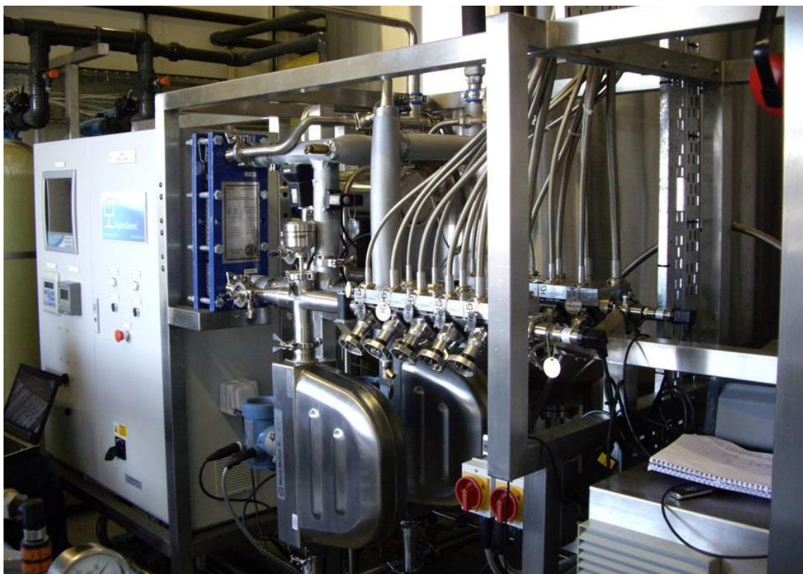
Figure 2 HydroGienic® skid at Dechra Pharmaceuticals showing connection of offtake hoses
